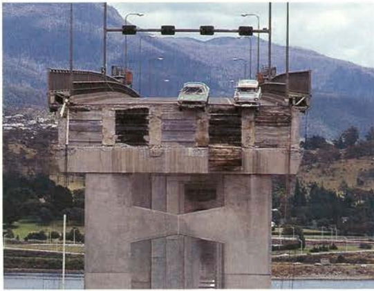
5 January 1975 The Tasman Bridge, Hobart, collapsed after being rammed by the freighter Lake Illawarra. The captain was suspended for six months and later that year retired. A Bailey bridge was opened further up the river to alleviate the delays to commuters.
